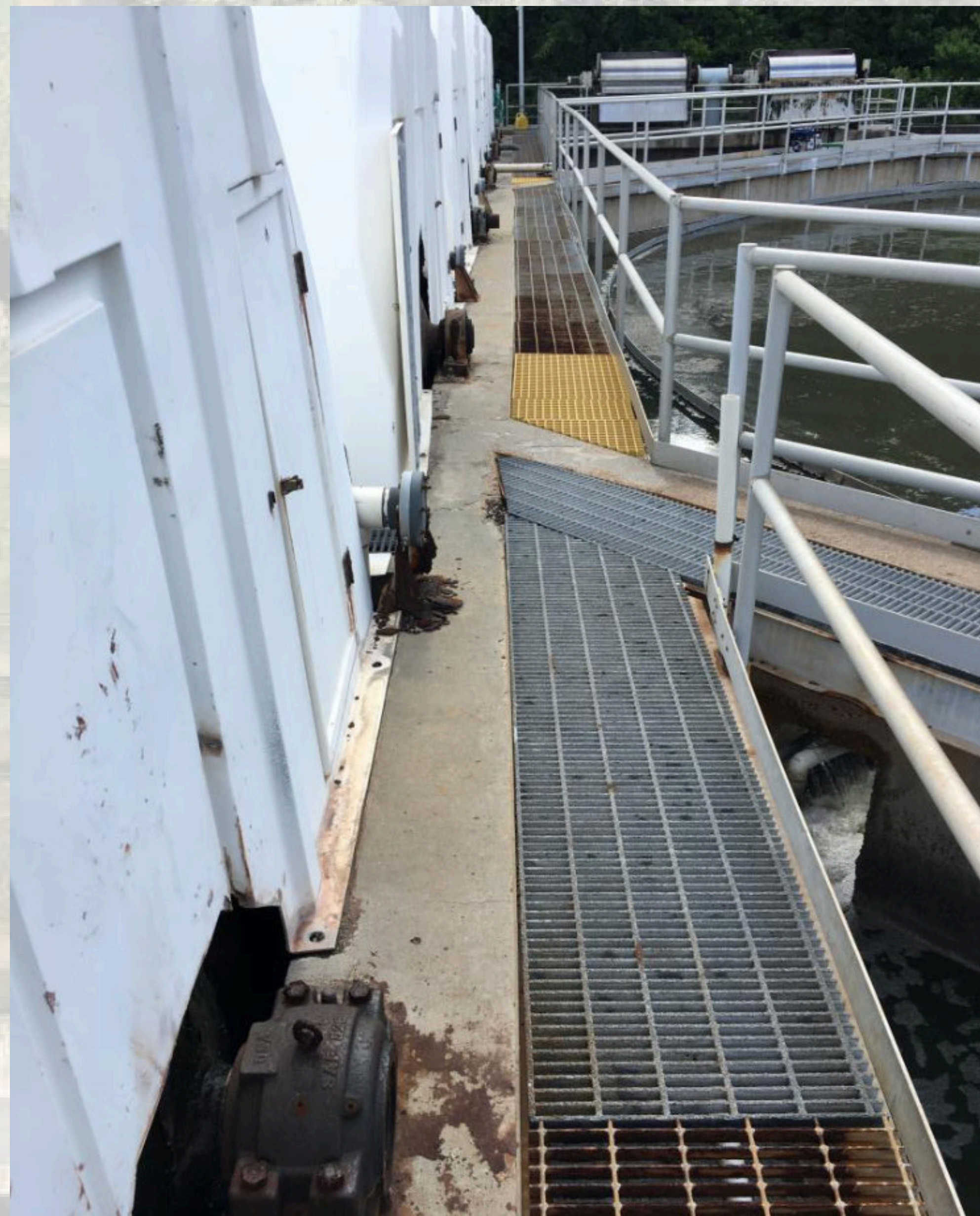
Exist RBCs (Corroded Bearings & Shafts)
