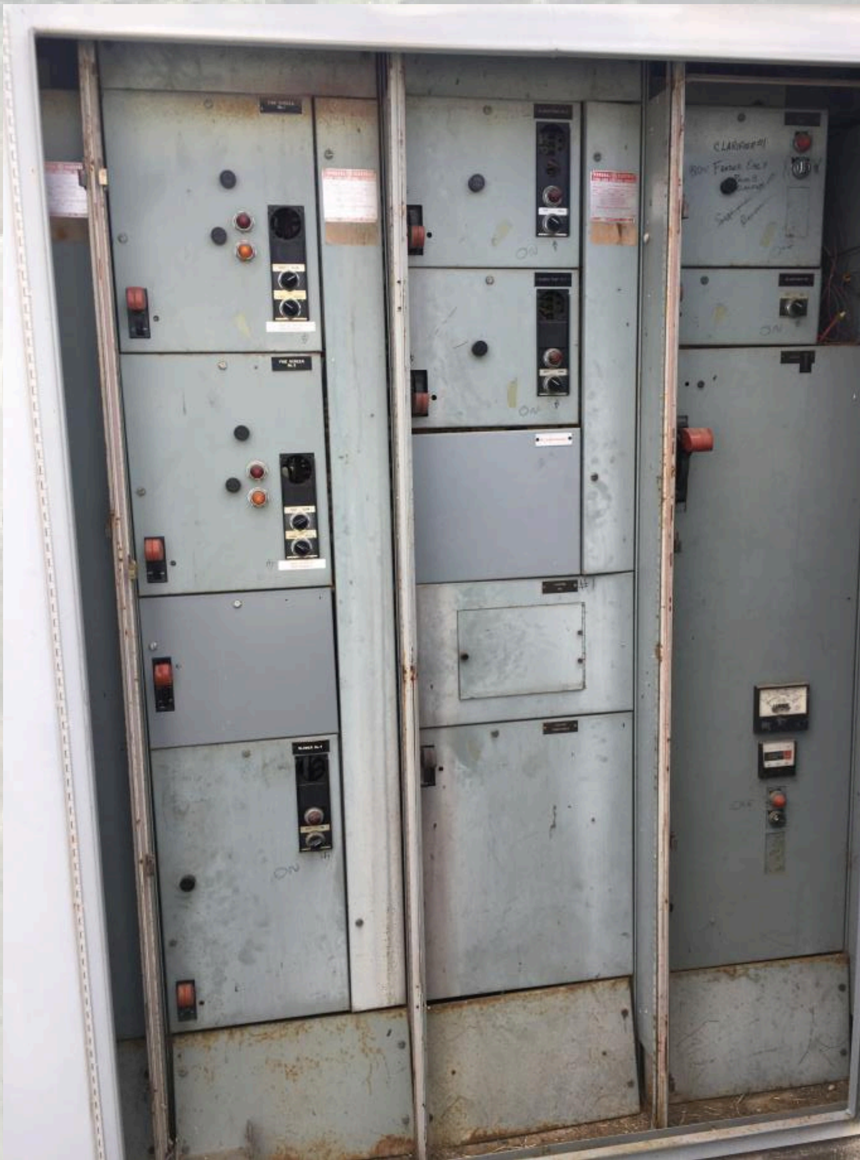
Exist MCC (Corroded, Outdated, & Unsafe)
