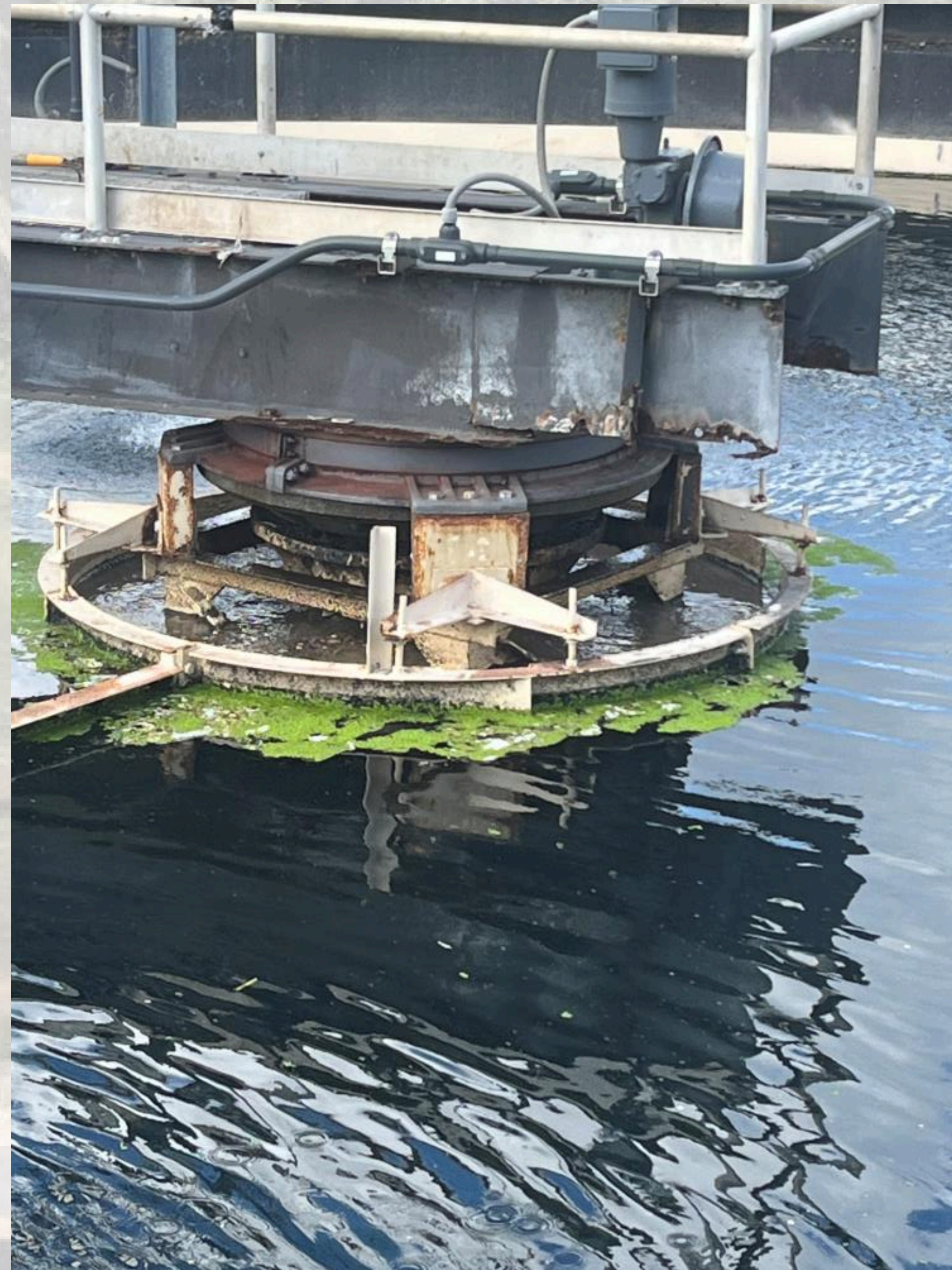
Exist Clarifier (Corroded Bridge & Mechanism)
