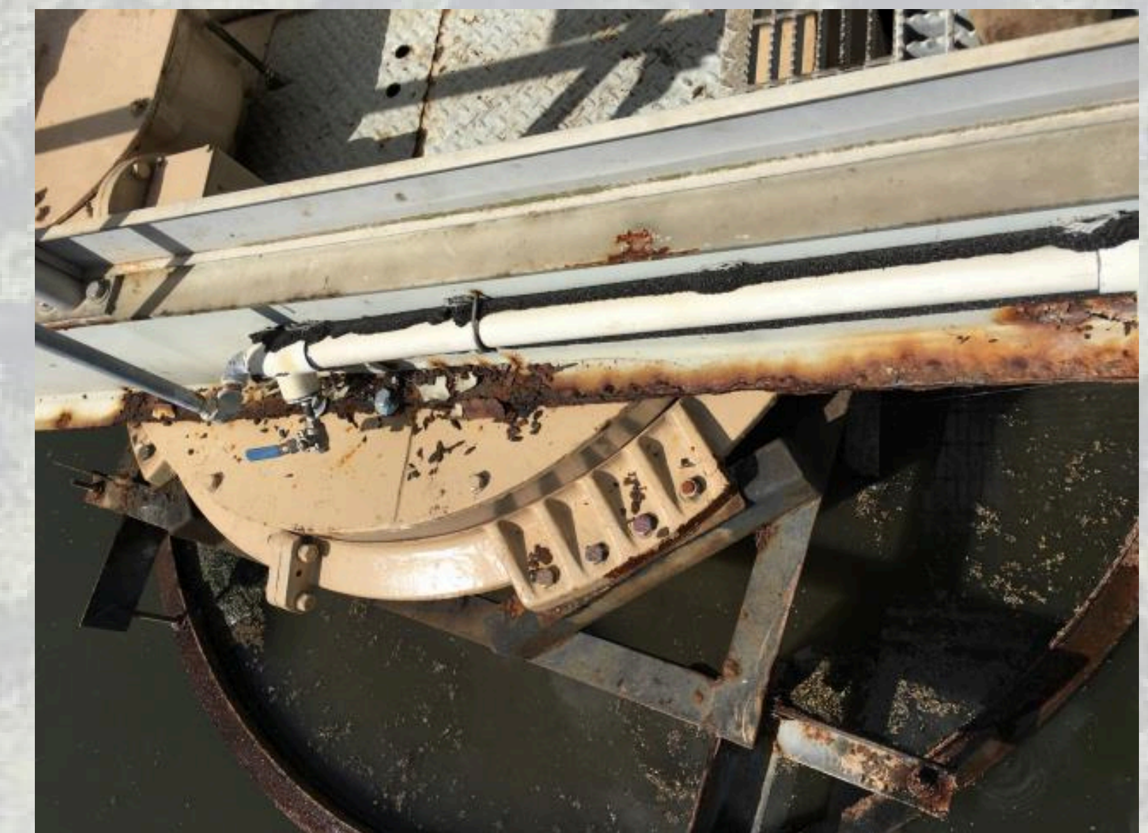
Exist Clarifier (Corroded Bridge & Mechanism)
